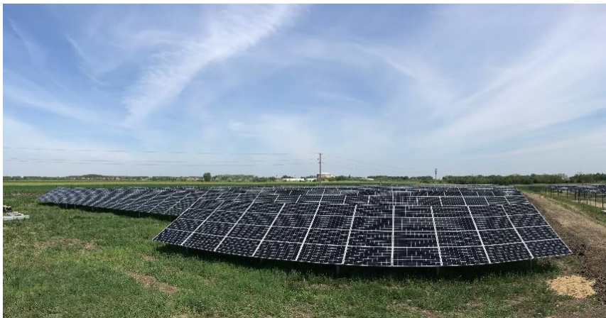
Image by Photon Energy: 1.4 MWp photovoltaic power plant in Kunszentmárton, Hungary.
