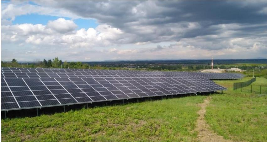
Image by Photon Energy: 2.1 MWp photovoltaic power plant in Mályi, Hungary.
