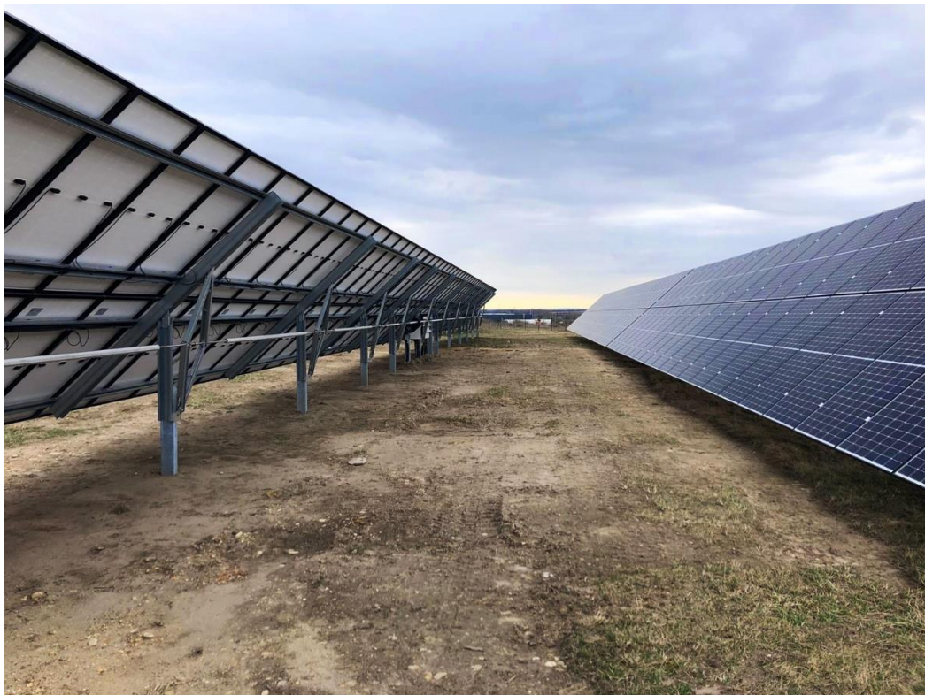
Image by Photon Energy: 5.4 MWp photovoltaic power plant in Tata, Hungary.
